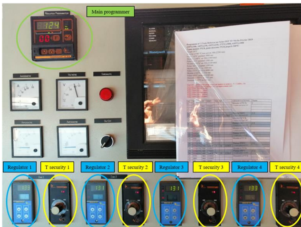
Figure A.4. Regulation system of the CEA oven based on a main programmer and four enslaved regulators controlling temperature variations in four different zones of the oven.
