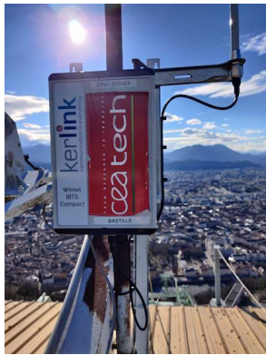
Fig. 19. Gateway BS_3 which is installed on the roof near the cable car station at Bastille, Grenoble
