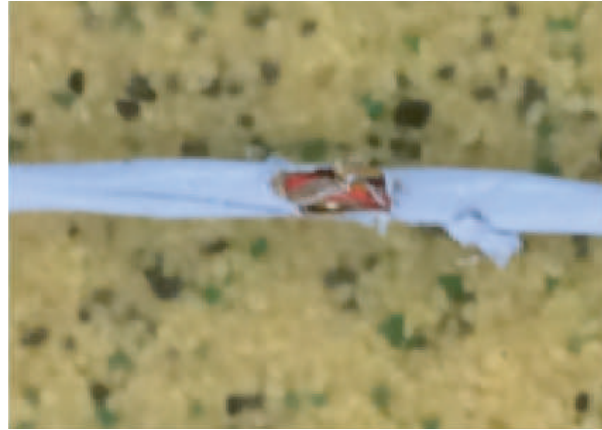
Figure 11: Shielding damage with width 5 mm at 10 m from the electronic board.
