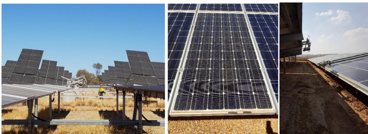
Figure 7: Left: Vegetation management of PV plant in Central Australia [2]; Middle: PV module (from a PV array in Central Australia) damaged during vegetation management due to pebbles [2]; Right: Automated cleaning of soiled PV modules in the Negev Desert, Israel [2].
