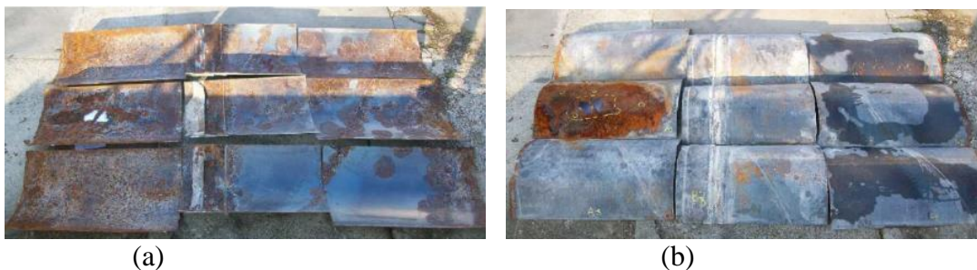
Figure 3: Pictures of corroded steel pieces, (a) inner side and (b) outer side
