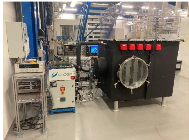
Fig. 1. ORC and boiling water tank
