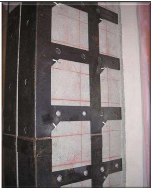
Strengthening and bonding after identifying the location of rebars in the concrete (red lines)
