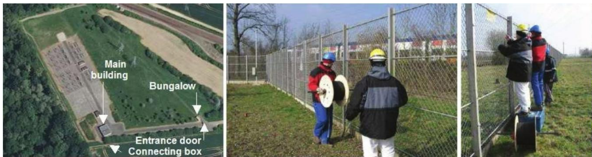
Figure 5. RTE electrical Substation (South-East of Paris, France) and sensing cable installation on fence
