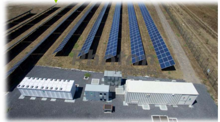
PV + Energy Storage System
