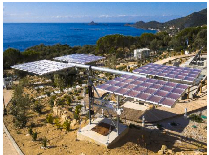
Fig. 3. The CPV system installed in Ajaccio.
