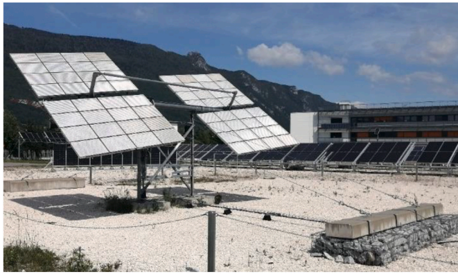
Fig. 2. CPV system installed in Le Bourget du Lac.
