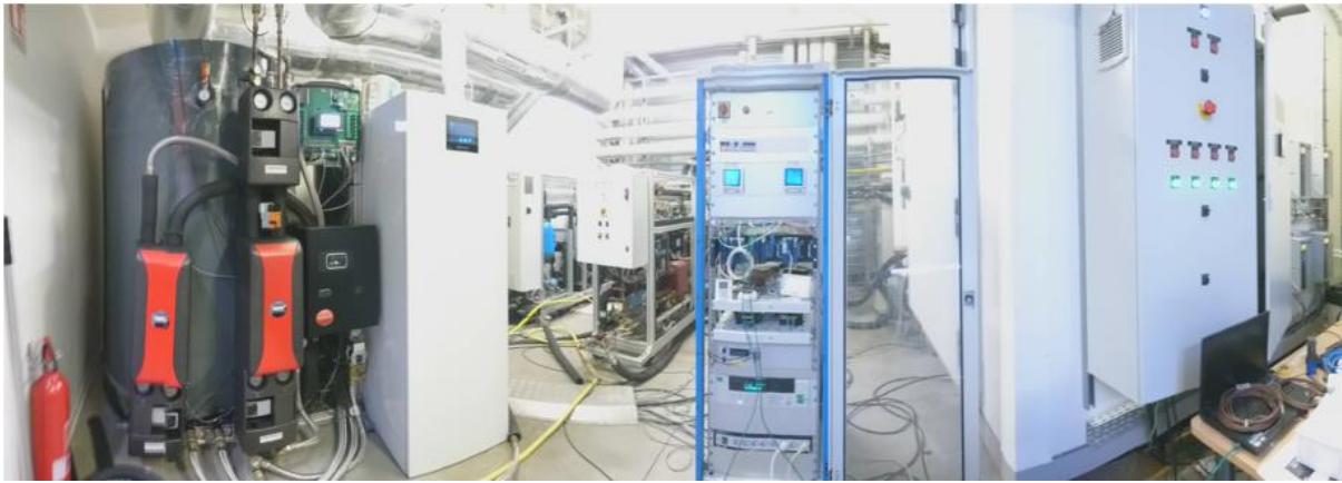
Fig. 4: HS2 concept and outlook of real prototype integrated in semi-virtual test bench
