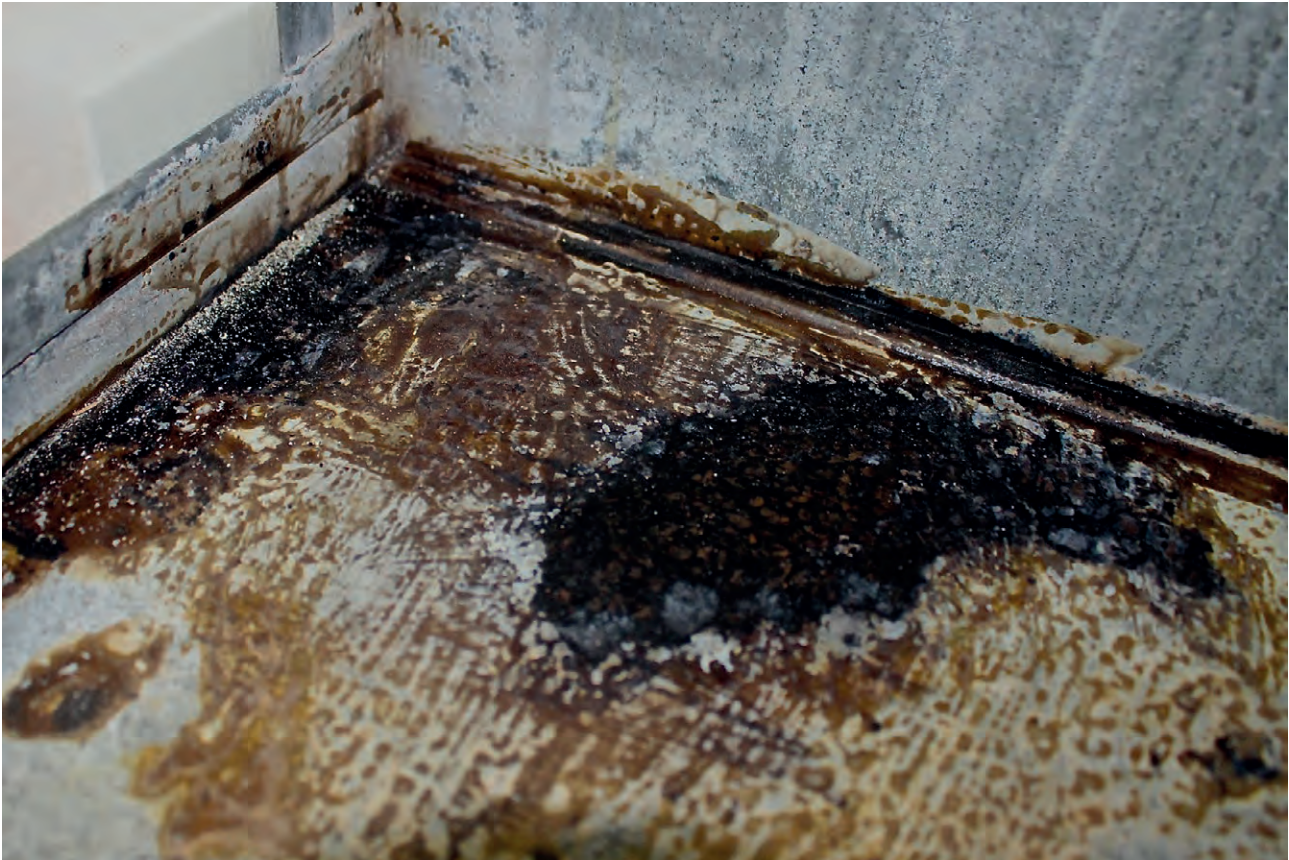
Figure 7 | Representative area of the brown/black crust on the bottom of the units. Photo by the author ©.
