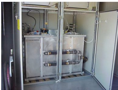
Fig. 4 +/- 30 kV 500A inverter for water purification (bacteria electroporation)
