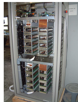
Fig. 6 High voltage inverter for plasma application
