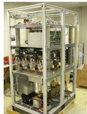
Fig. 2: Power Electronics Cabinet
