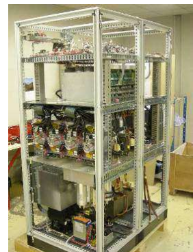
Fig. 2: Power Electronics Cabinet
