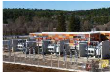
63kV / 15kV substation
