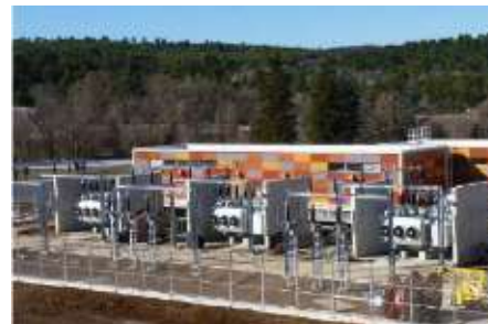
63kV / 15kV substation
