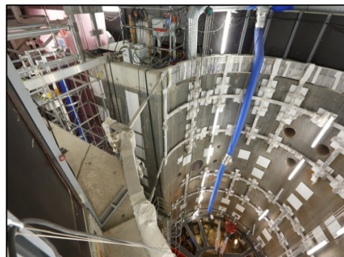
April 2014: Reactor pool internal structures © CEA
