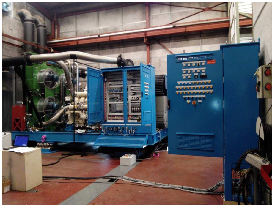
In-factory tests for emergency diesel generators (End 2014)
