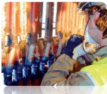
Repair of stress corrosion cracking in an ultra- supercritical (USC) power plant, from Laborelec Suez, 2013, http://www.laborelec.be/ENG/publications/newsletters/newsletter-2013-june-power-generation/how-to-repair-potential-cracks-in-t24-material/
