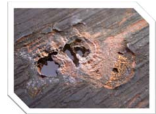
Pitting corrosion of an oil tank
