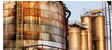
Atmospheric corrosion in a chemical plant
