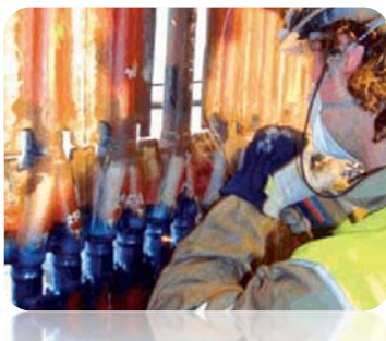
Repair of stress corrosion cracking in an ultra- supercritical (USC) power plant, from Laborelec Suez, 2013, http://www.laborelec.be/ENG/publications/newsletters/newsletter-2013-june-power-generation/how-to-repair-potential-cracks-in-t24-material/
