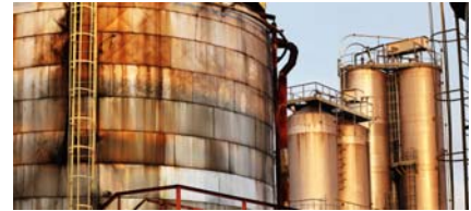
Atmospheric corrosion in a chemical plant
