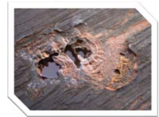
Pitting corrosion of an oil tank
