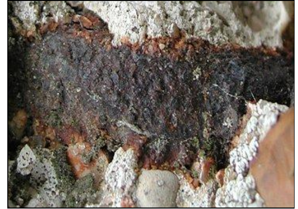
Corroded steel rebars in concrete structure
