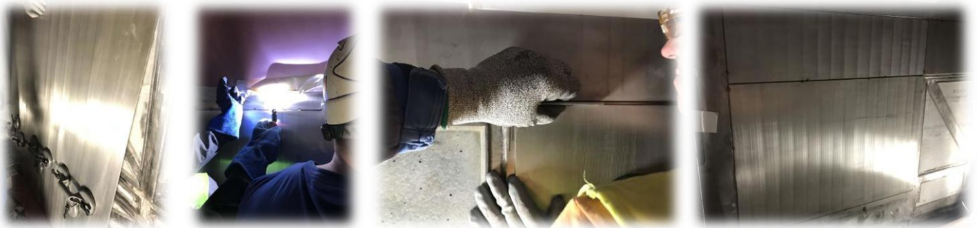
Fig. 1: Hot cells liner
