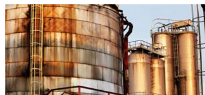
Atmospheric corrosion in a chemical plant
