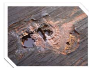
Pitting corrosion of an oil tank
