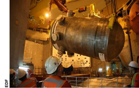
PWR (EPR) reactor pressure vessel
