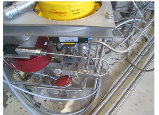
Fig. 3. View of the throttle valve in the MEXIICO installation.
