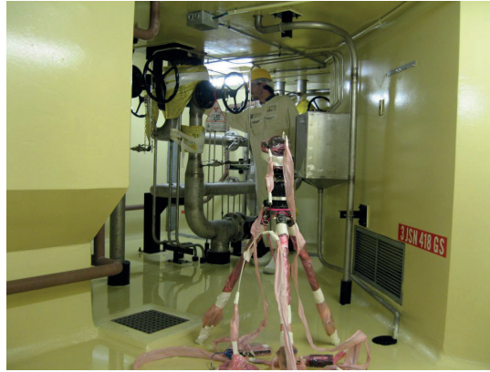
Figure 4.1 – Observation du point chaud par la caméra gamma (locaux du BAN). Observation of the hot spot by the camera (nuclear auxiliary building).
