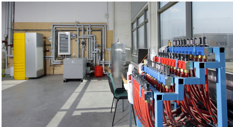
Figure 5: View of operating installation - CLIPSOL's SCS, absorption chiller, cold storage tank and ground loop collector in the technical area
