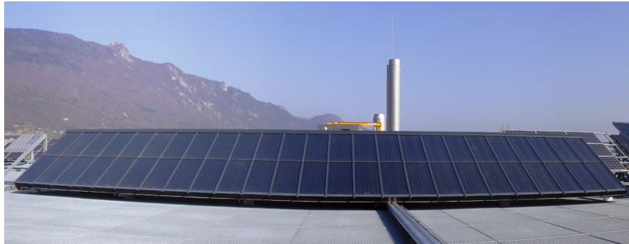
Figure 3: 30m 2 flat plate solar collector field on the top roof
