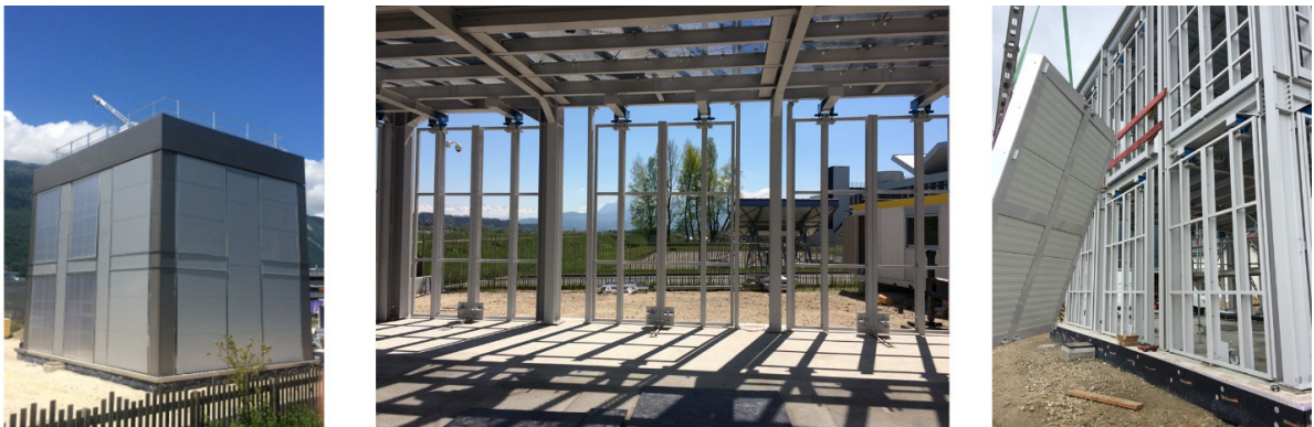
Fig. 3. FACT during the building phase. External view (left), the secondary structure (center) and façade installation (right).
