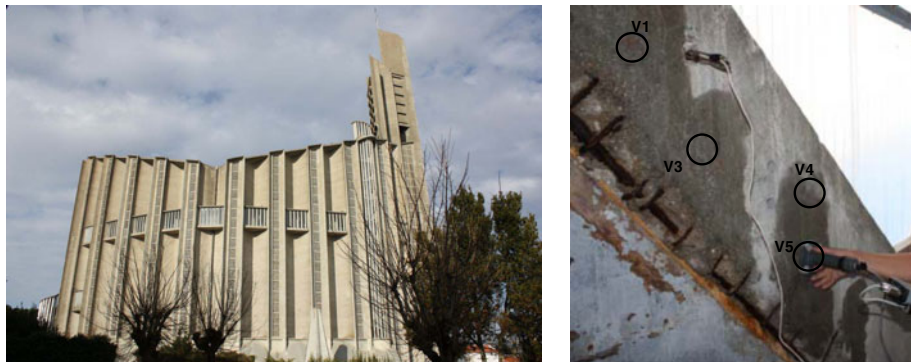
Figure 15. Royan cathedral and intensity corrosion measurement.
