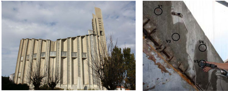
Figure 15. Royan cathedral and intensity corrosion measurement.
