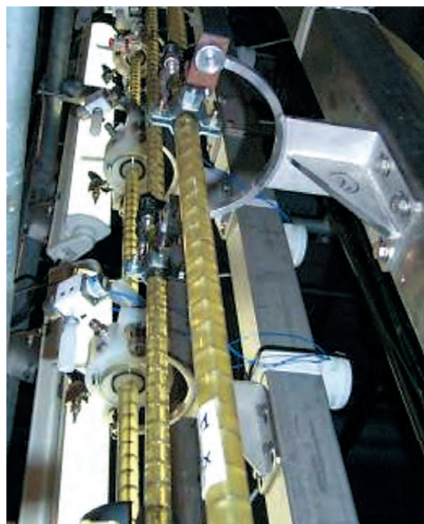
Fig. 132. A view of the pulsed columns, set up in the shielded process line (CBP) in the ATALANTE facility, for the purposes of the technical feasibility demonstration tests for enhanced partitioning, carried out in 2005.
