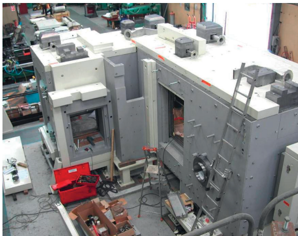
Fig 84. Construction of shielded cells for the VERDON experimental device at the STAR underground laboratory.
