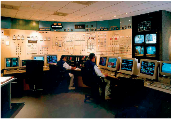
Fig. 68. OSIRIS control room.
