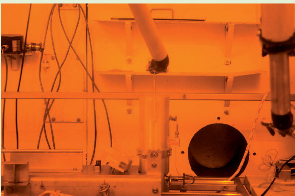
Fig. 76. The MOSAÏC calorimeter for measuring residual power in shielded cells.
